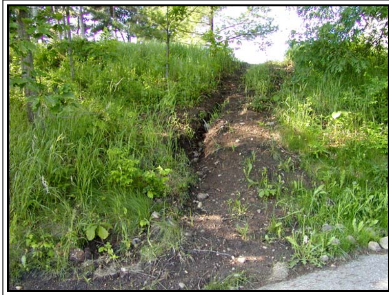
Figure 1 – Unstable slope behind tennis court
