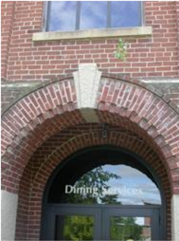
Fig. 2. Cottonwood tree seedling growing out of the brick above the entrance to the Refectory.
