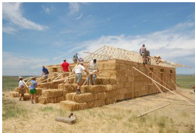
Figure 2: A straw bale home under construction demonstrates the building method of bale stacking for wall construction.
